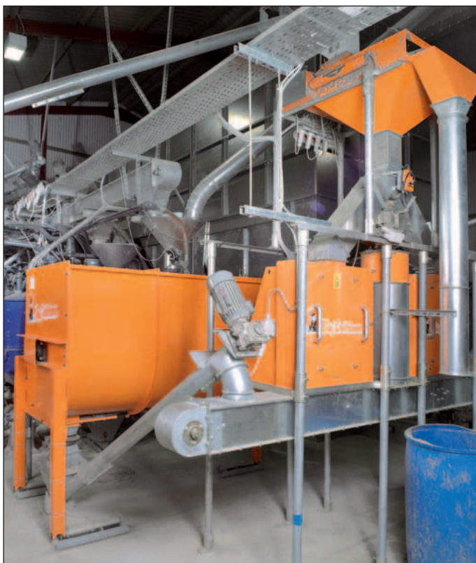
Feed kitchen with feed mill, mixer and HYDROMIX
